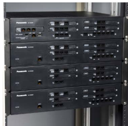
in 19 inch rack
